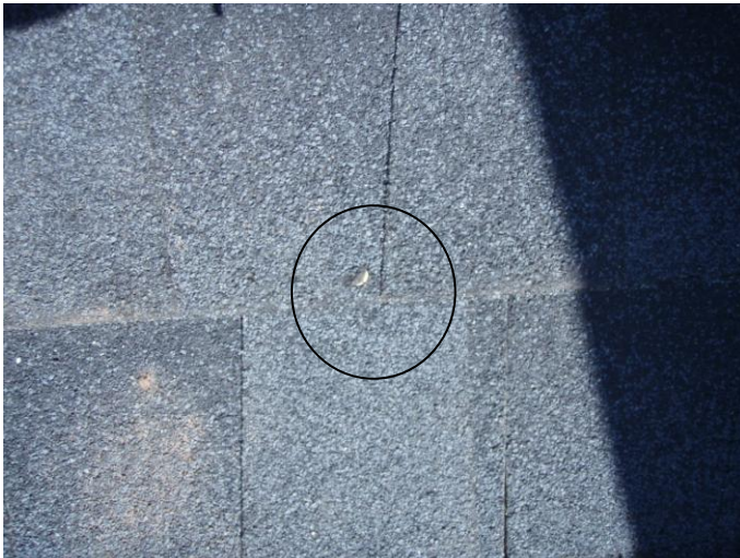
10. Nail pops, low nails and holes in shingles
