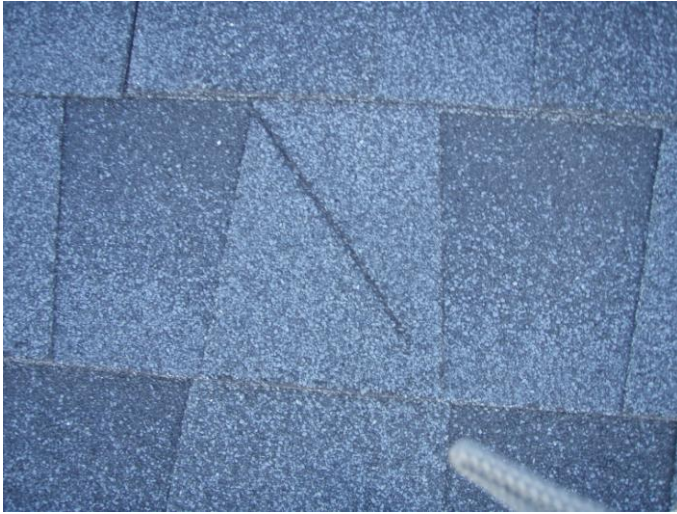
7. Shingles have several blade marks from cutting shingles during installation.
